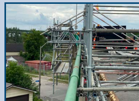
Scaffolding for the bridge railings HRCSA paint project, 2022 (Photo: Courtesy of IBA)
