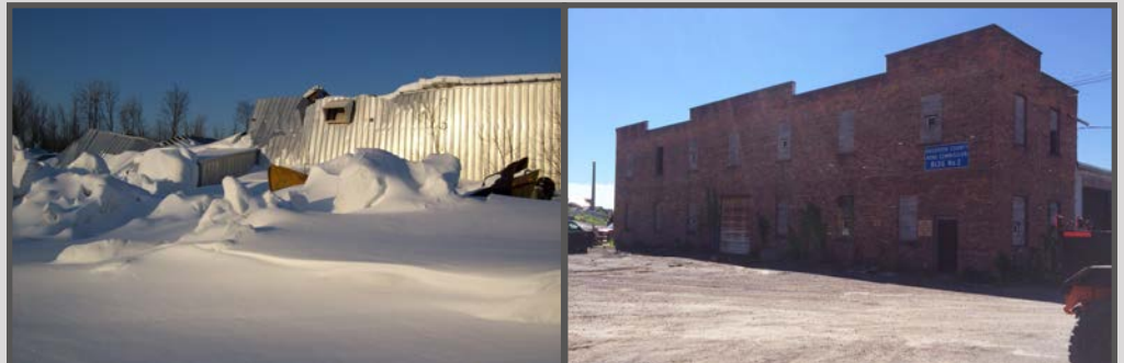
Houghton CRC’s old facilities – Left: Cold storage after roof collapse in 2013; Right: Original 100-year-old maintenance shop (Photos: Courtesy of Houghton CRC)
