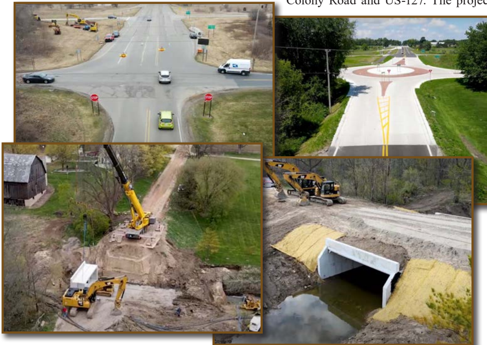
Two of the three projects Trotter assumed when he took over as director of engineering at Clinton County Road Commission; top left and right - Dewitt & Clark roundabout project; bottom left and right - Church Road bridge replacement (photos courtesy of Clinton County Road Commission)
