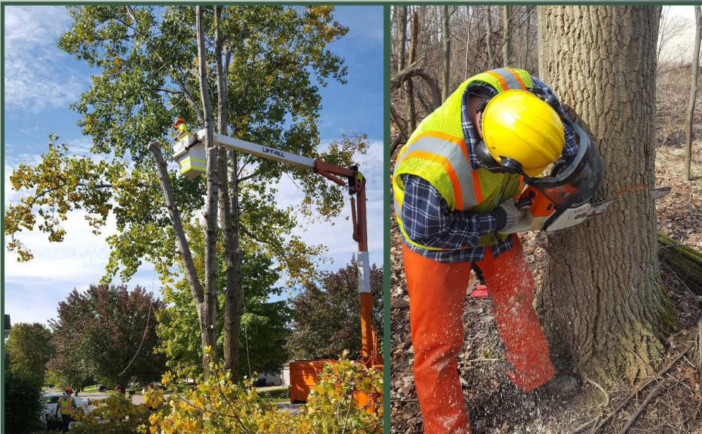
Left: Tree cutting operation using ropes to guide the fall; right: notching a tree using a chainsaw (Photos courtesy of Dustin Brighton)
