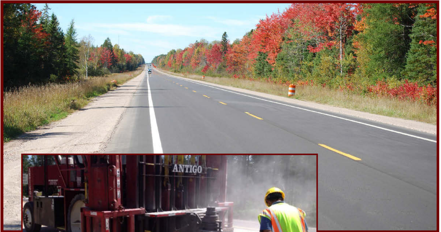
Rubblization project on M-28 near Raco, Michigan. Top: completed project; bottom: rubblization in progress (Photos courtesy of the Michigan Department of Transportation)
