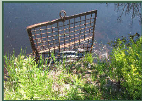
Culvert guard (Photo: CTT Archive)
