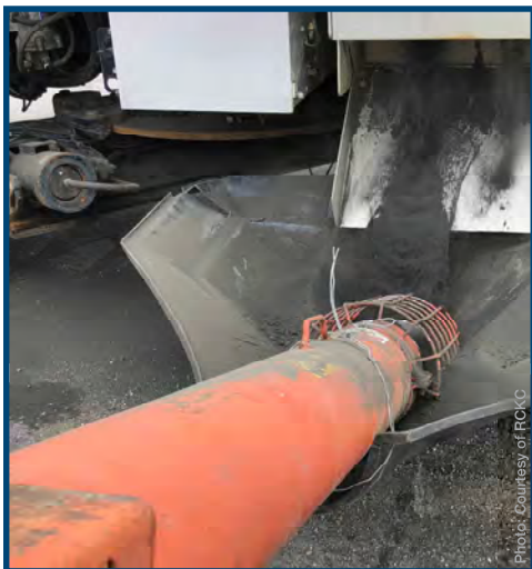
Rubber granules passing through the auger conveyor for loading into the asphalt distributor
