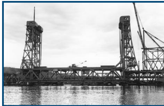
Construction of the Portage Lake Lift Bridge, Houghton/Hancock, Michigan. Photographer unknown. Photo courtesy of Michigan Tech Archives.
