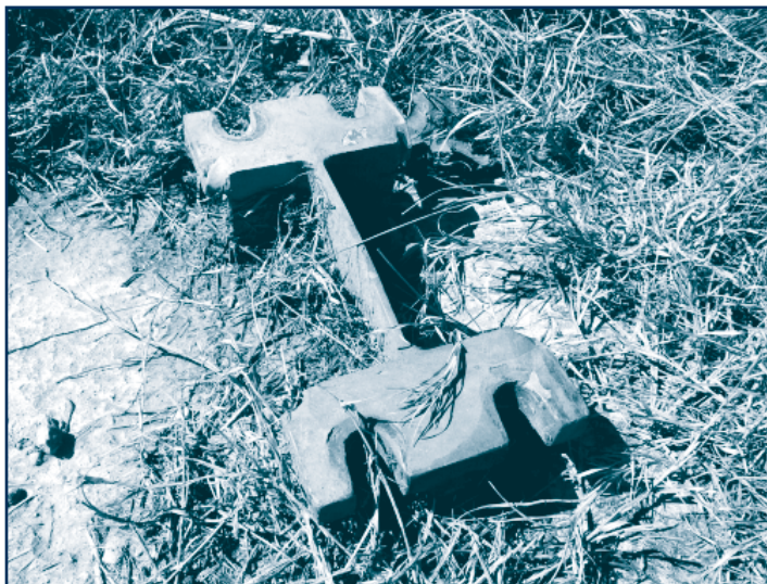
The in-ground traffic sign base, left after the sign broke away in the crash.
