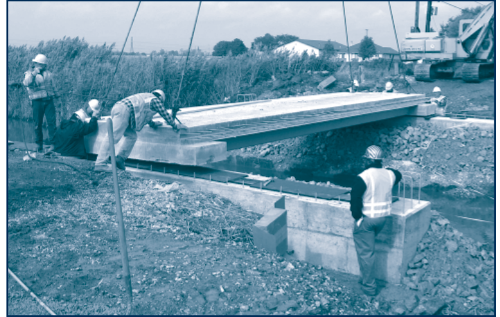
Monroe County Road Commission maintenance workers place a prefabricated deck slab for the new Suder Ave. Bridge.
